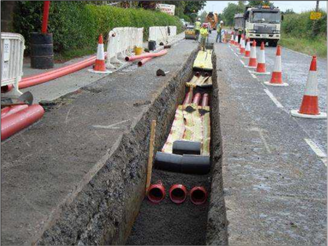
Figure 2-3: Typical 220 kV installation.
